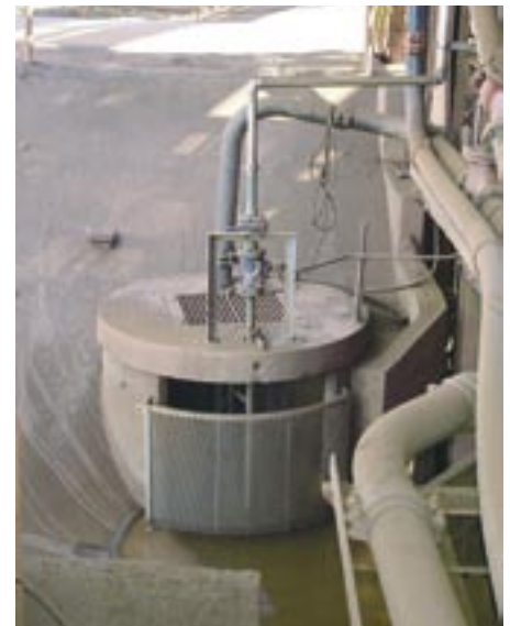
The optimum pump sump with the removable screen that makes cleaning simple
