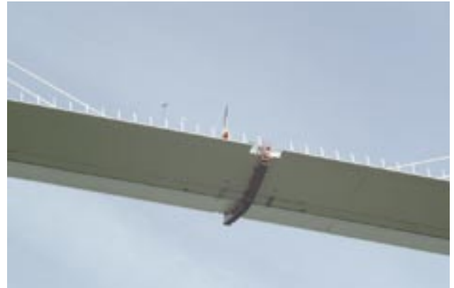
Final Hydraulic Launch Successfully Closes last Gap in the Millau Viaduct in the South of France. The job is done.
